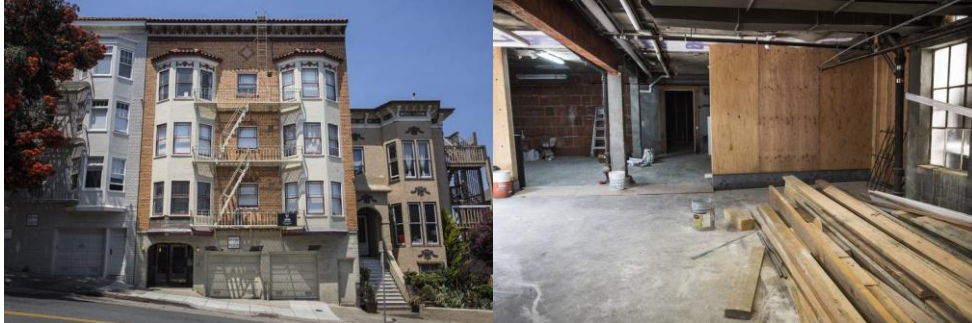
The basement of a three-story building being renovated for housing units in San Francisco.
